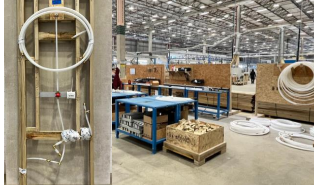
2. Shaft assembly station and hydraulic kit
