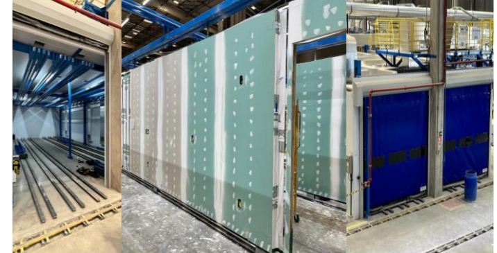
3. Panel caulking station and drying chamber
